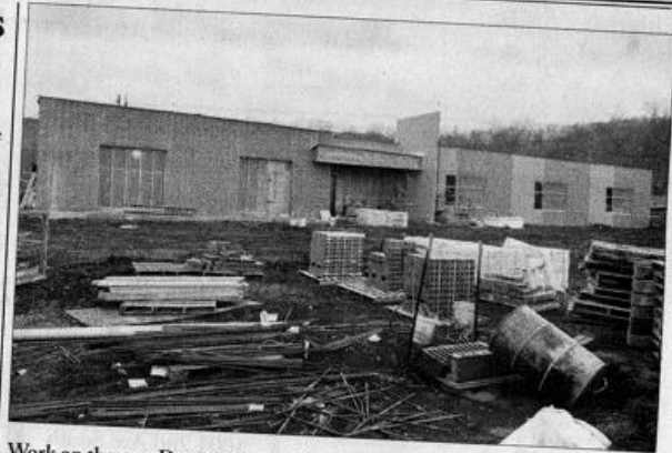
Work on the new Denison Career Academy facility will be finished in time for fall classes. Submitted photo
